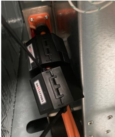
(a) Ferrite cores on cables in the cabinet of a product
